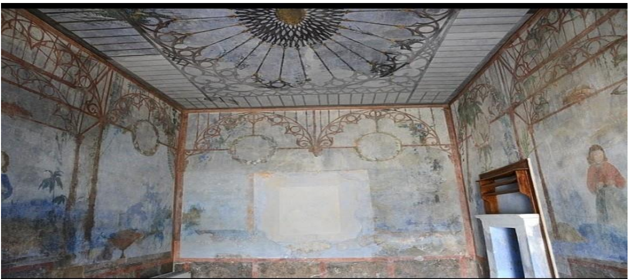
Figure 1. The wall paintings of Four Seasons inside the N. Gyzis building. (left) The representation of Summer. (right) The representation of Spring. (center) The damaged wall painting of Winter.
